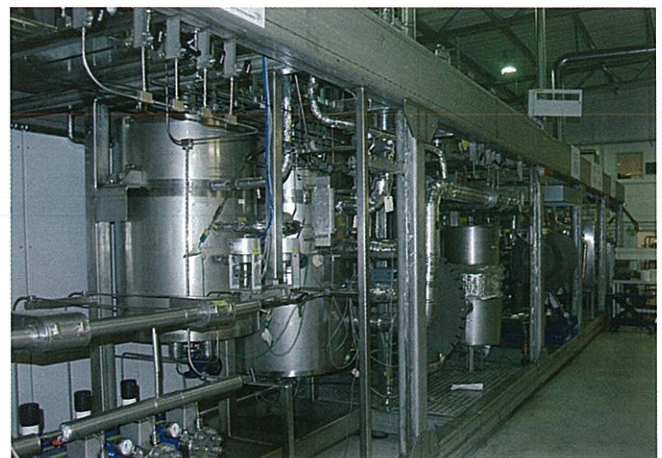
Demo plant, Copenhagen Denmark
